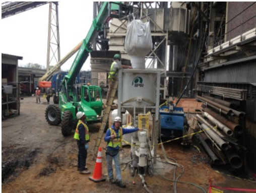
A 54” cooling line, lying beneath this IPR Industrial EcoCast crew, was leaking into a 13,500 kV room shown on the right side of this photo.
