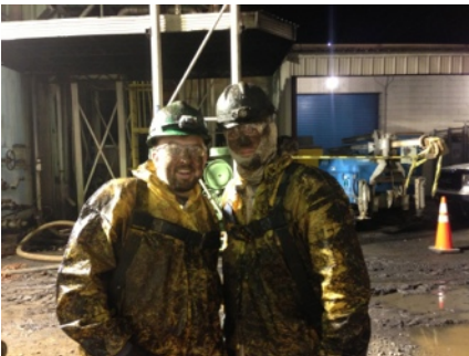
IPR Industrial personnel worked round the clock, in shifts, to complete the cleaning, prepping, and restoration of the leaking 320 ft. cooling line.
