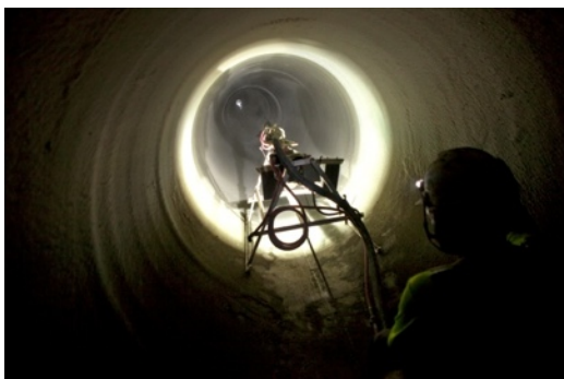
The EcoCast system was lowered into the deteriorated 320 ft. line from a man-way and relined it with a structural and corrosion resistant geopolymer. The line renewal took only 3 days to complete.
