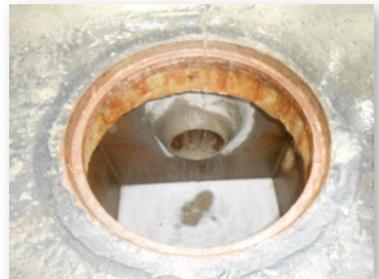
One of several hundred leeching and deteriorated manholes discovered at an oil refinery.
